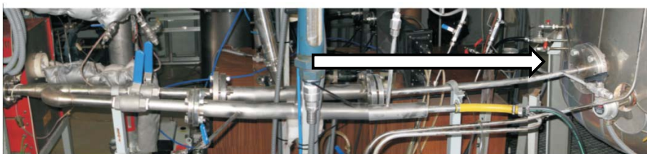
Fig. 10 Injection line entering into the PECA-vessel
