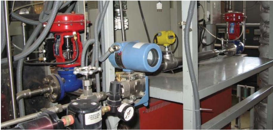
Fig. 11 Control valves (pressure and gas mass flow rate) of the injection line
