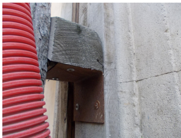
Fig. 18 _ Level of corrosion D of a bracket that has not been protected with paint
