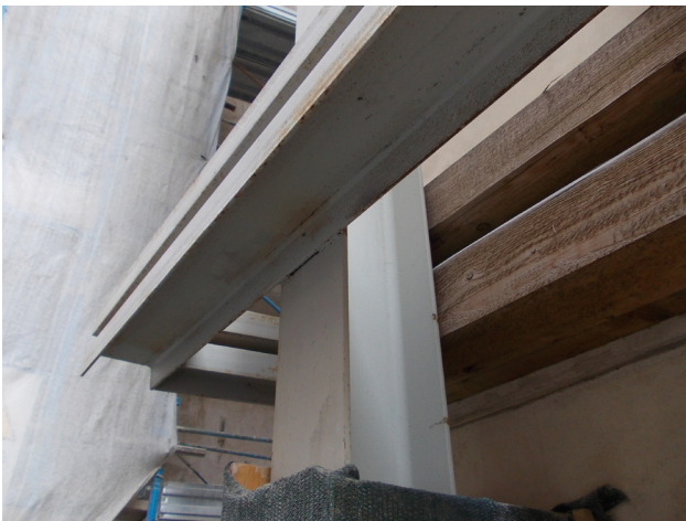
Fig. 14 _ Uprights- Rusting degree R0-R2 Crossbeams- Rusting degree R3
