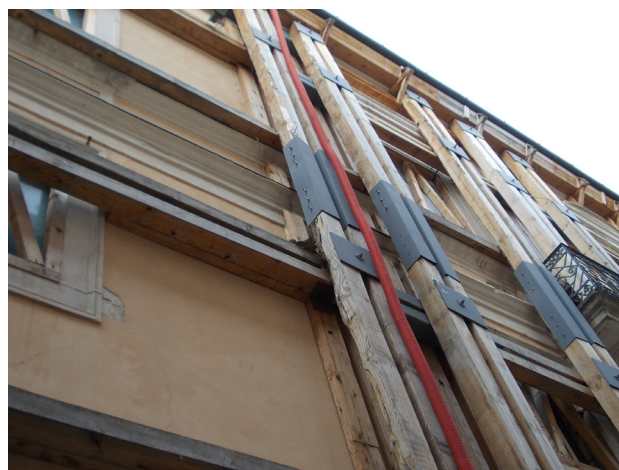
Fig. 12 _ Connection between uprights and crossbeams through U steel bolted elements- High reversibility.
