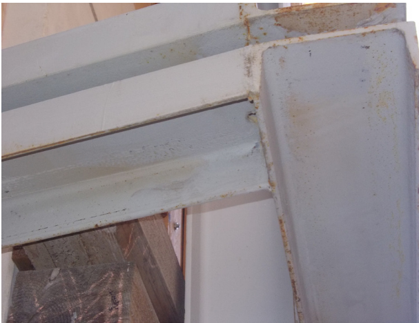
Fig. 13 _Corner. Rusting degree R4-R5
