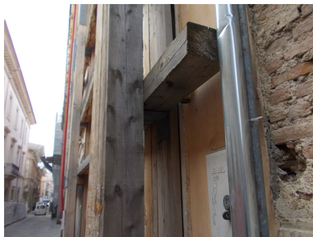
Fig. 16 _Discoloration of the elements
