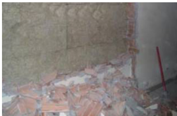
Fig.10 _ Centro Porretta Terme. Within some walls, glass fibre insulation is present, which was not seen in the survey carried out in the preliminary phase.
