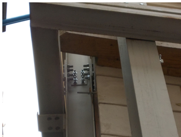
Fig. 10 _ Connection between uprights and crossbeams by bolting. High reversibility. Connection between uprights and crossbeams by welding. Low reversibility.
