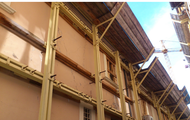
Fig. 30 _ Uprights and cross beams with UPN profiles coupled on the side of the web plate
