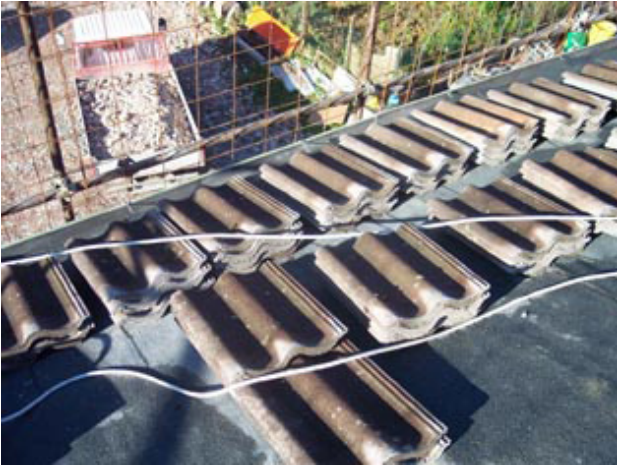
Fig. 13 _ Centro Porretta Terme. Removal of the roof covering, which is necessary to isolate and waterproof the roof. The tiles are stacked on the roof and then reassembled.
