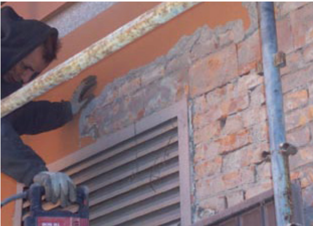
Fig. 14 _ Centro Porretta Terme. Removal of plaster on the outer portion of the wall, where the building expansion was made.
