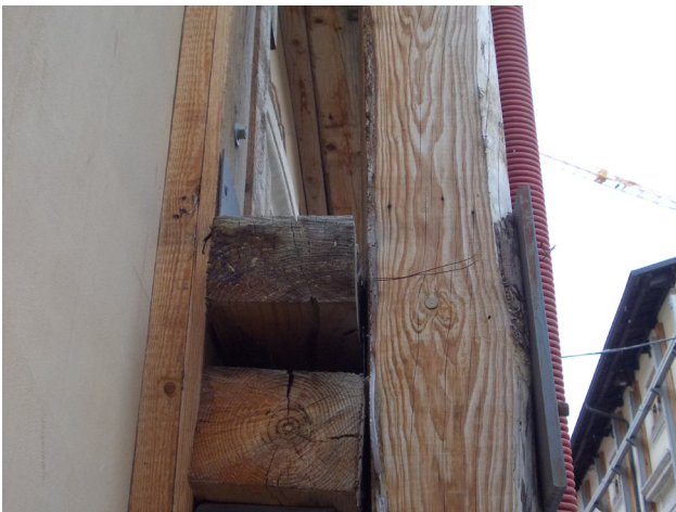
Fig. 20 _ Connection of uprights and crossbeams and radial fissuring of the elements
