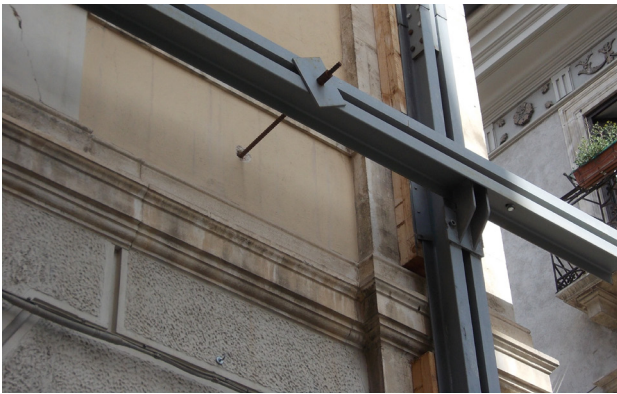
Fig. 28 _Uprights and crossbeam with UPN profiles coupled on the site of web plate, steel shelf
