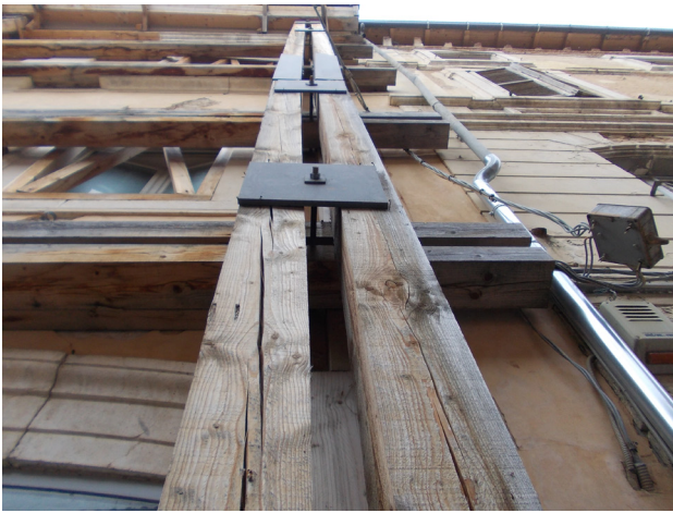
Fig. 19 _ Degradation with fissuring of the uprights, chromatic alteration of the terminal part of the crossbeams
