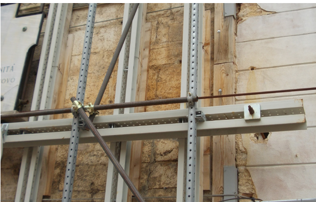
Fig. 31 _Uprights and cross beams with UPN profiles coupled on the side of the web plate, steel shelf, upwinds with tubes-clamps system
