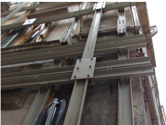
Fig. 29 _Uprights single UPN profiles, crossbeams with UPN coupled profiles, steel shelf, single UPN beams
