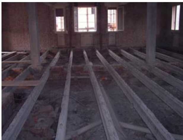
Fig. 12 _ Centro Porretta Terme. Reuse of the joists in the new horizontal structure
