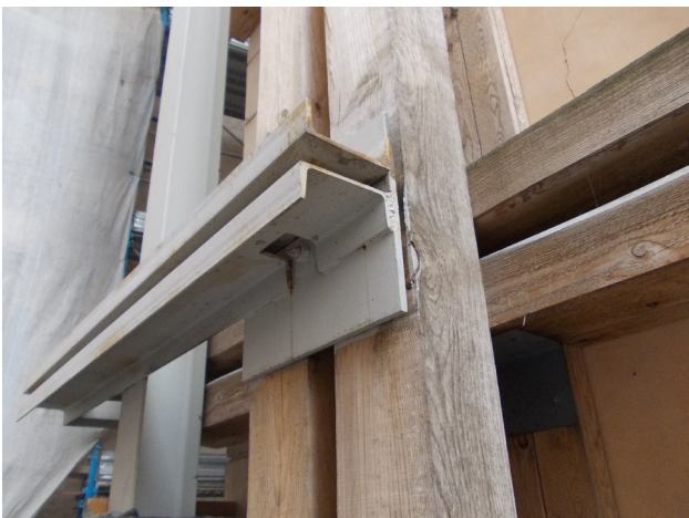
Fig. 15 _ Final part of crossbeams- Rusting degree R4
