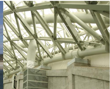
Figure 16 Isolation bearings at Hiraga dome
