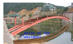
Fig 2 Failure of the bridge
