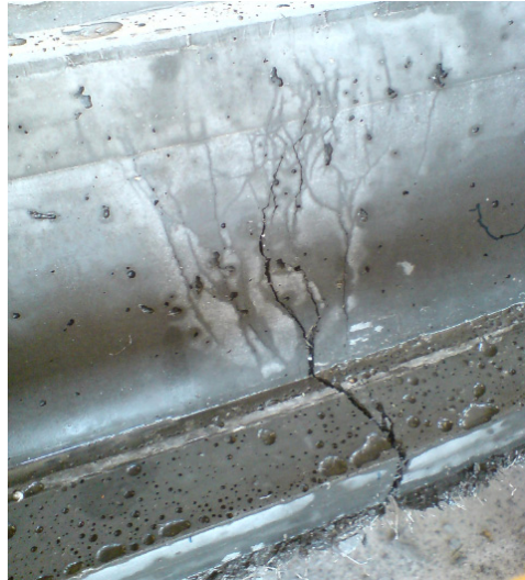
Figure 16. Crack pattern around the principal crack at rupture time.
