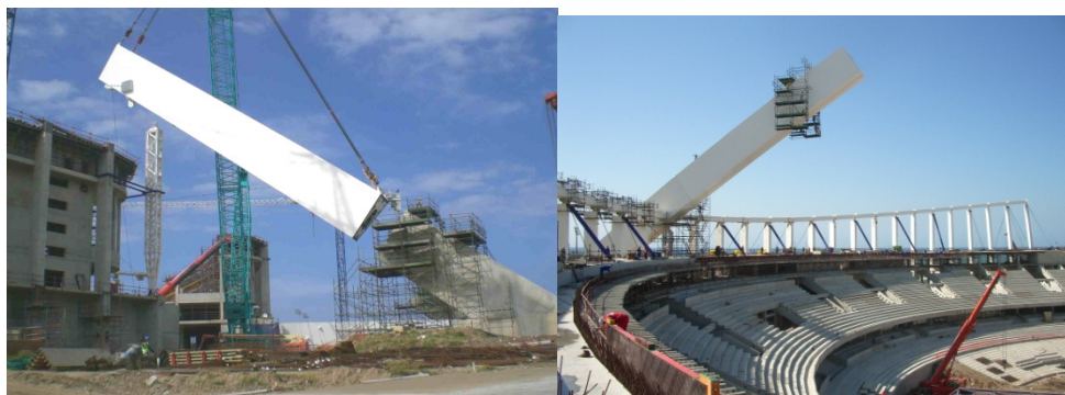
Figure 13. Big lift of first four arch elements and accurate positioning onto supports
