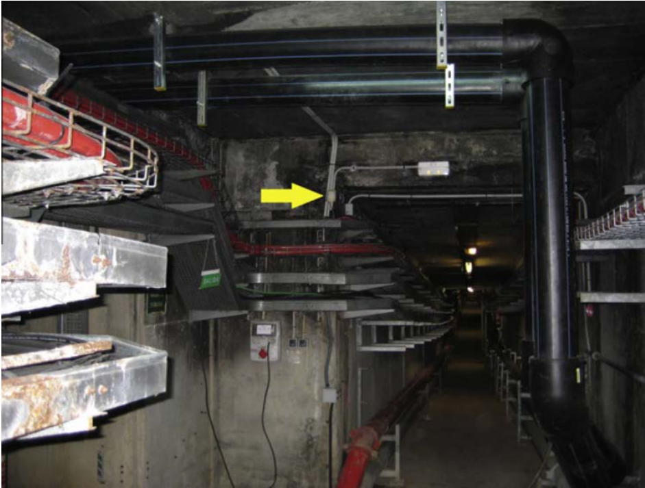
Figure 2. Some sensors are intentionally visible while others are hidden. The petty intruder will be detected by visible sensors, while covert sensors will deal with the professional criminals or terrorist.
