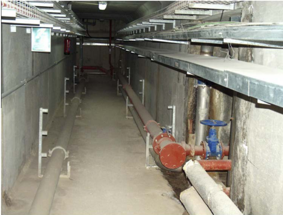
Figure 1. Walk-through utility tunnel cross-section permits the installation, maintenance and removal of utilities without making street cuts or excavations. Pipe and conduit racks are mounted on the utility tunnel walls, improving accessibility and maintainability, and minimising personal injuries.
