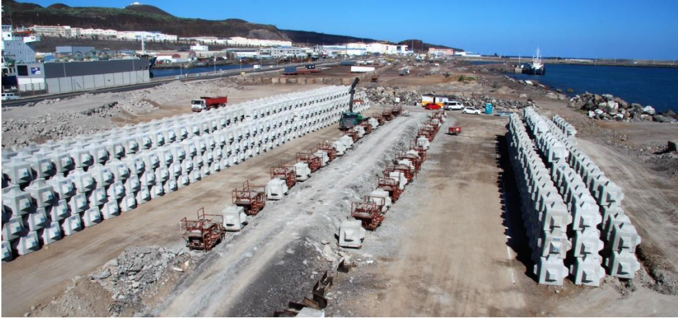
Figure 5.9 Block yard and production line of 6-tonne ( 2.6 \text{ m}^3 ) Cubipods (Port of Las Palmas, Spain).
