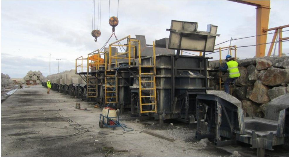
Figure 5.7 Molds and production line of 25-tonne (10.6 m 3 ) Cubipods (Port of Punta Langosteira, Spain).
