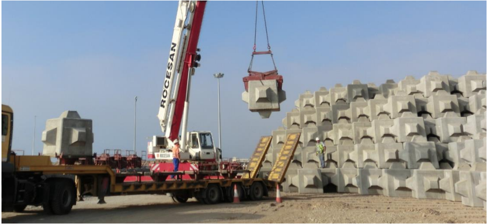
Figure 5.14 Loading Cubipods onto a platform to be transported to the placement site.
