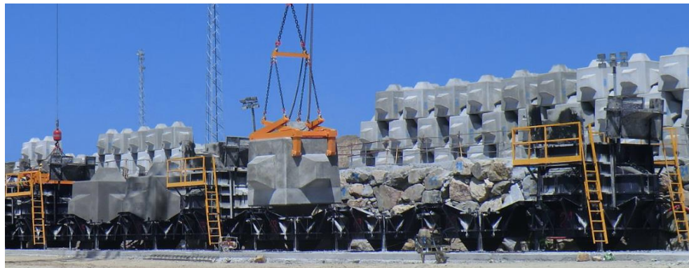
Figure 5.1 Vertical molds and bases to manufacture 45-tonne (19 m 3 ) Cubipod® units (Port of Punta Langosteira, Spain).
