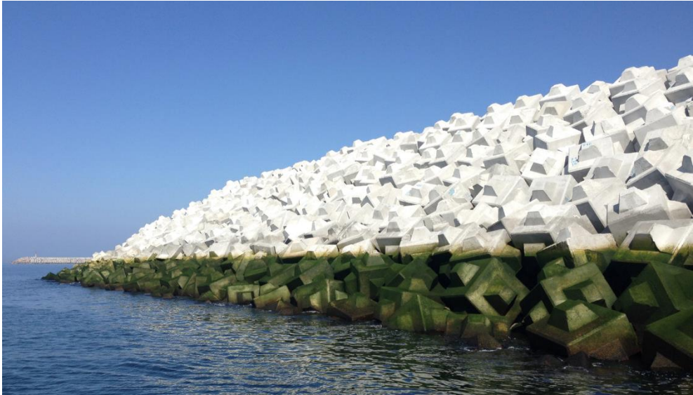
Figure 1.2 Twenty five-tonne Cubipod ® units in the Western Breakwater of the Outer Port of A Coruña at Punta Langosteira (Spain).
