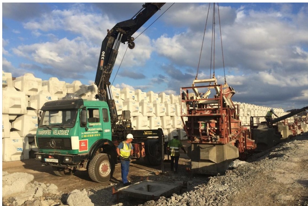
Figure 5.8 Vertical molds and bases to manufacture 6-tonne (2.6 m 3 ) Cubipod ® units (Port of Las Palmas, Spain).
