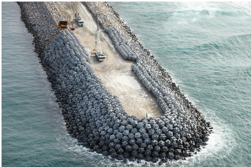
Figure 6.1 Twenty-five-tonne single-layer Cubipod® armor protecting the Southern Breakwater at Punta Langosteira (A Coruña, Spain).
