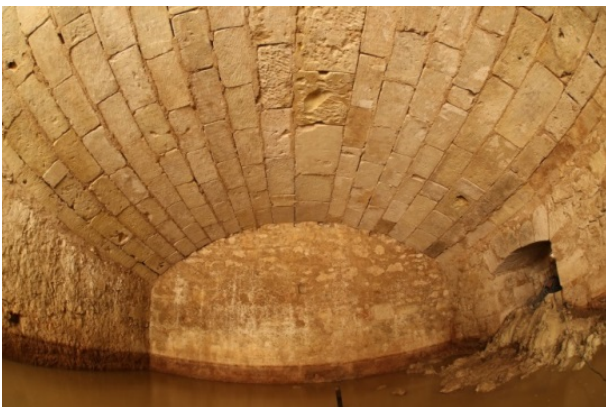
Figure 2: Image of the second room of the latrine, captured with a fisheye lens and with opposite lightning.
