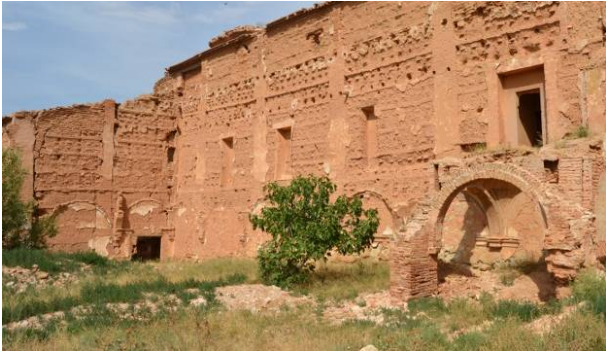
Figure 6: Cloister current aspect (2015). The remains of the arches of the vaulted gallery can be seen on the wall.
