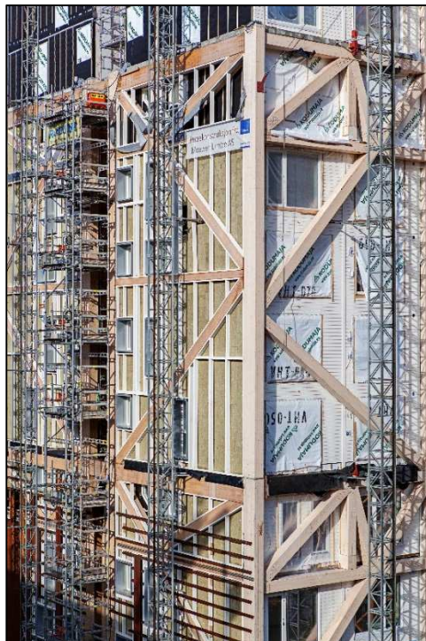
19. Picture of the construction. The timber-frame and the modules after its installation – source: ARTEC
