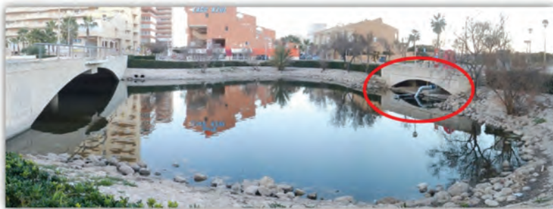
Figure 4: Infrastructure for pumping water towards the sea.
