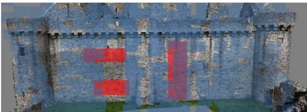
Figure 5: Camera locations (in blue) for the acquisition of data with the PG-2 system. The three areas of the wall used for the performance assessment are shown in red.
