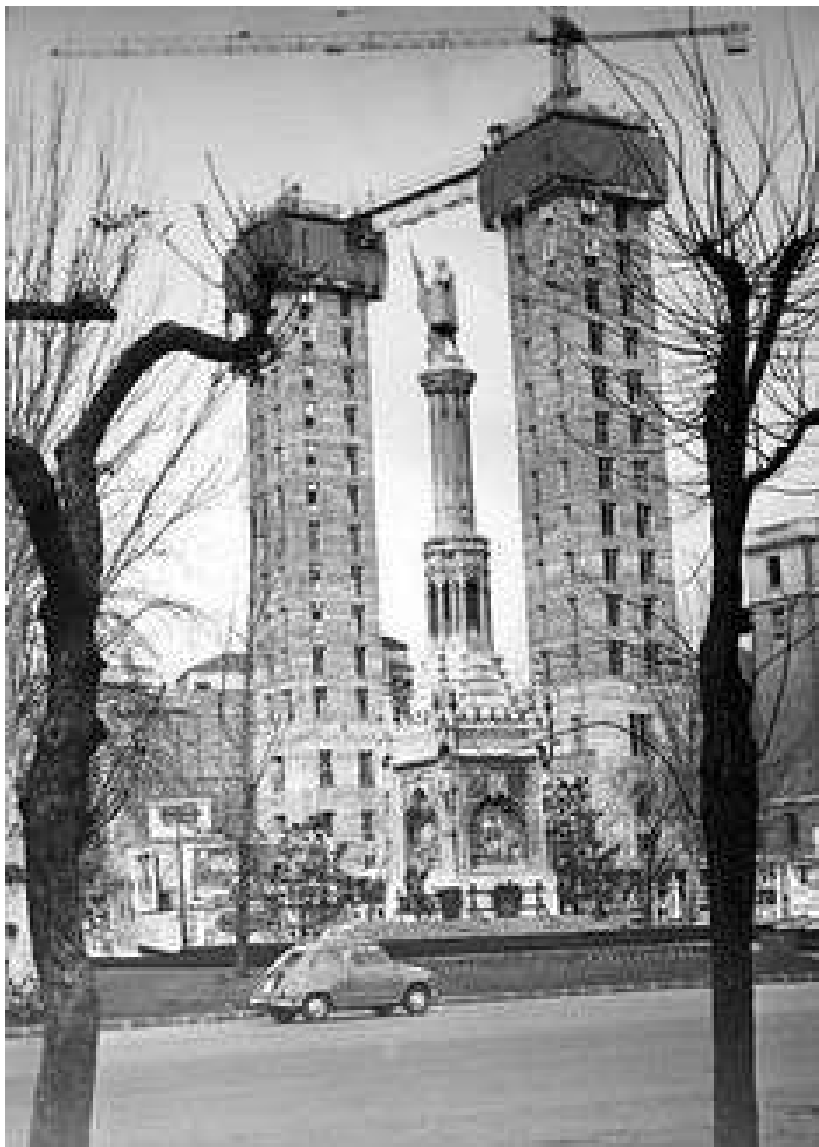
39. The system of execution of the central nucleus of the tower will be realized with doublé formwork of small height.
