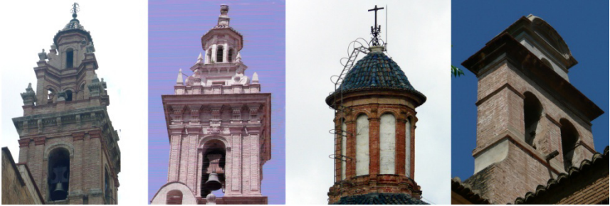
Figure 7: Bell Towers with gauged brickworks: San Esteban Church , Royal College Seminar Corpus Cristhi , Royal Basilica and St. Ursula church examples (Cristini; Ruiz-Checa).
