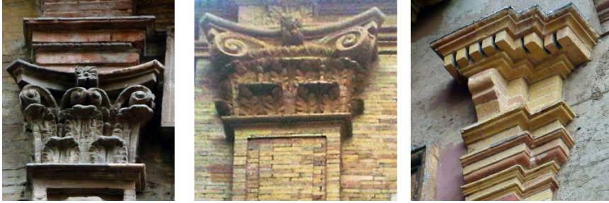
Figure 4: Scrolled volutes and capitals with “marly” bricks: Condes de Alpuentes Palace, Communion Chapel in St Martin Church, Royal Basilica, Valencia (Cristini; Ruiz-Checa).
