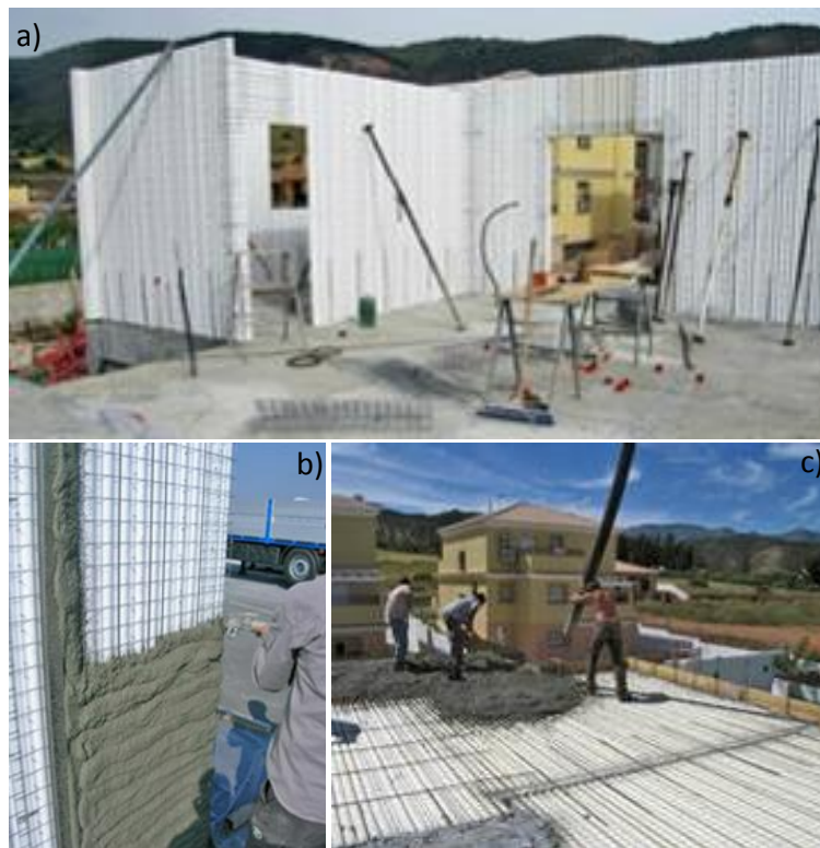
Fig. 10 MSP Construction system (a) Assembly of panels (b) Shotcrete sprayed on walls. (c) Concrete pouring on floor slabs.
