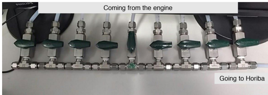
Figure 3.6. Rail and valves for intake gas measurement selection.
